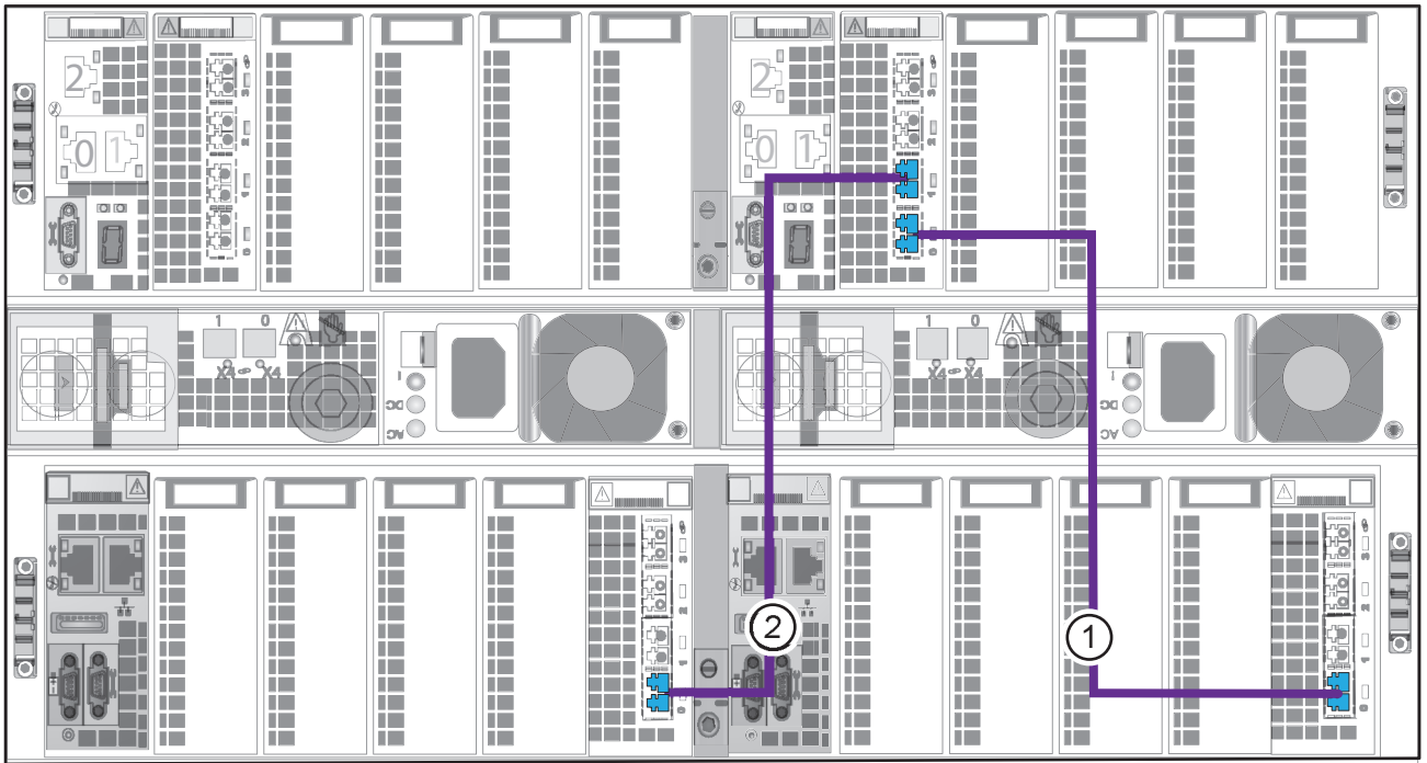
Figure 32 Cable storage processors to blade enclosure 0
