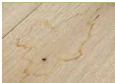
Ugly water marks can quickly appear due to insufficient resistance against liquids.
