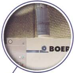
Central exhaust hood Zentralabsaughaube
