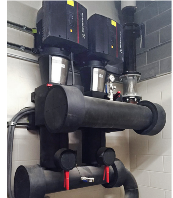
Wall hung CRE-H model pumps in hot and chilled water system
