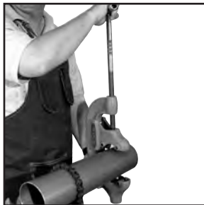
Figure 1: Cut tube to desired length using a tube cutter
