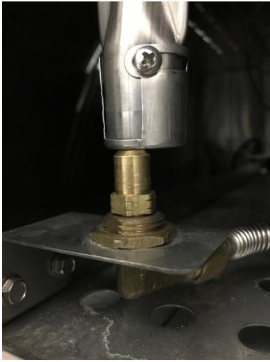
REAR BURNER NOT PROPERLY SEATED
