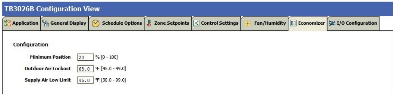
Fig. 40. Economizer Screen (AHU)
