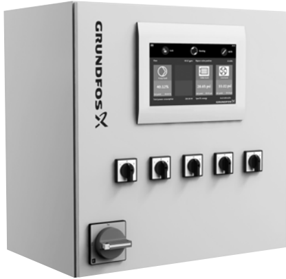
Fig. 4 Front panel of the main cabinet
