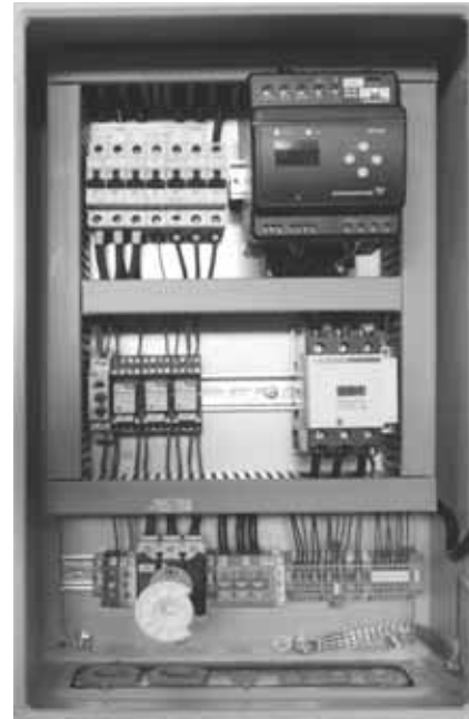
Fig. 13 Inside view of MP 204 panel
